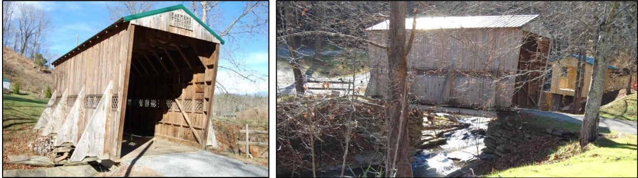
Figure 45: Covered bridge [D] – at left, looking north from Farmers Fish Camp Road; at right, looking south toward creek and road with covered deck [E] at right
